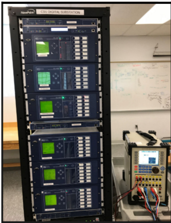
Figure 7 Hardware Installation of IEDs in Rack and Test Set
